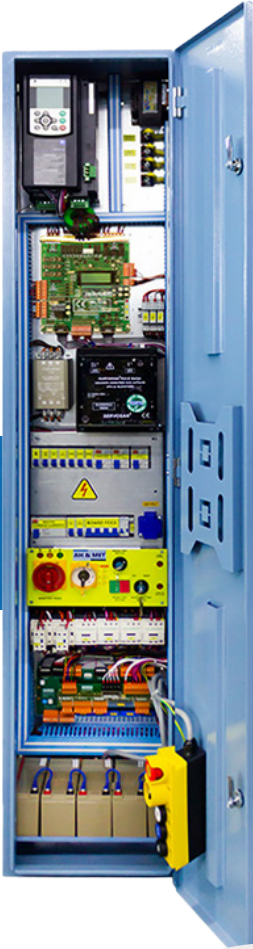
Fuji ml50s Kontrol Paneli Fuji ml50s Control Panel
